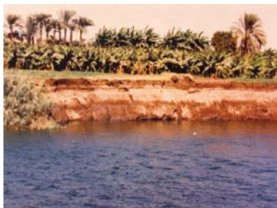
Photo 2: land erosion due to seepage effect
